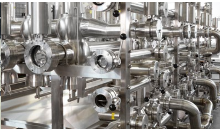
← Fully automated fermentation / storage with the piping system SOL
